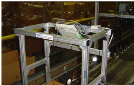
Open Frame Structure Single Antenna Overhead
